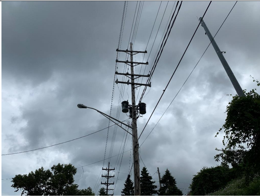
Photo 9: Looking east towards 3 pole transformer.
