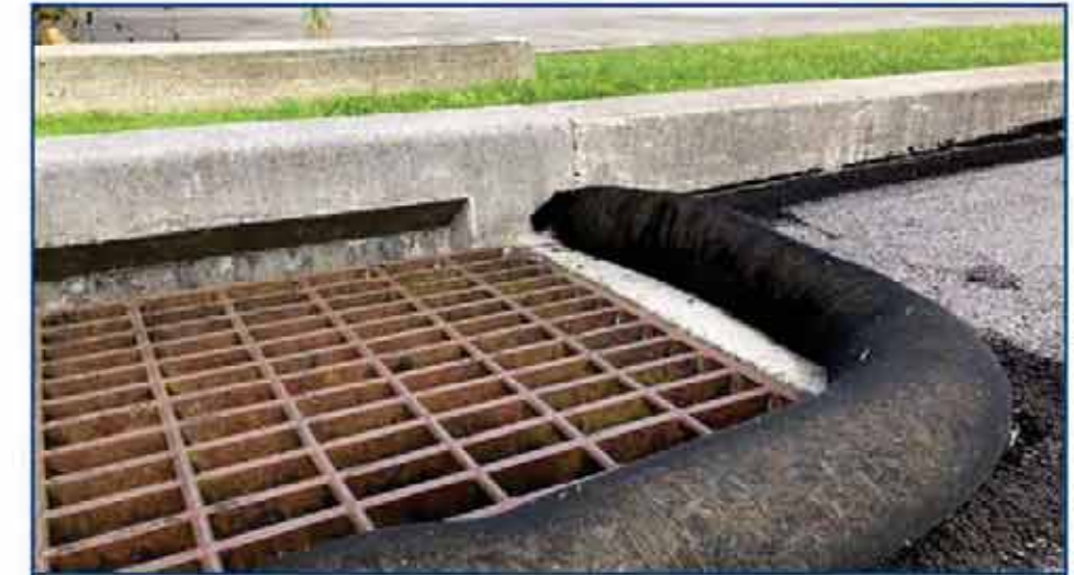
Devices such as compost filter socks are placed during construction to prevent sediment from reaching waterways.
