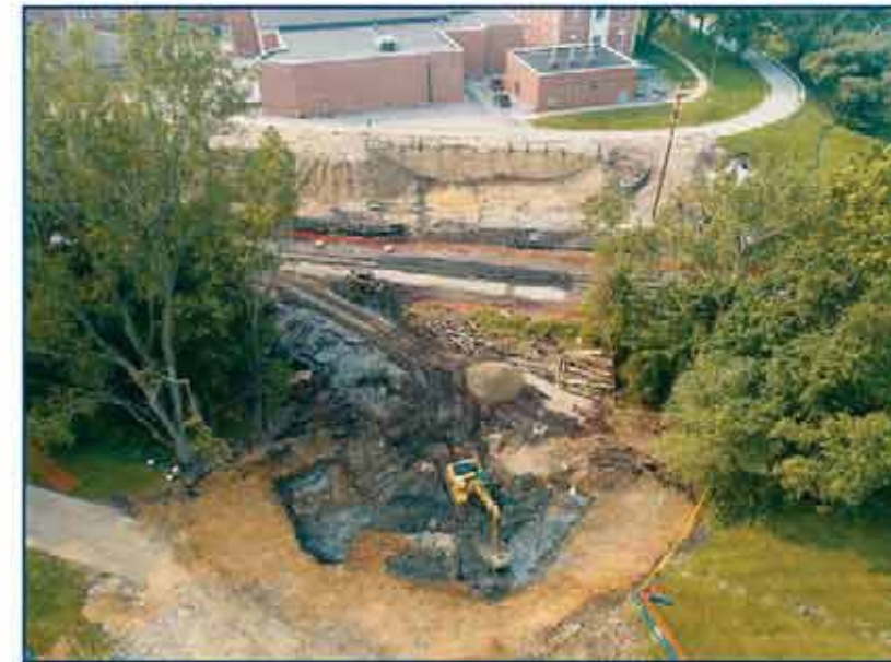
Construction of a new bridge over the railroad tracks is underway at the Soldiers' & Sailors' Home.
