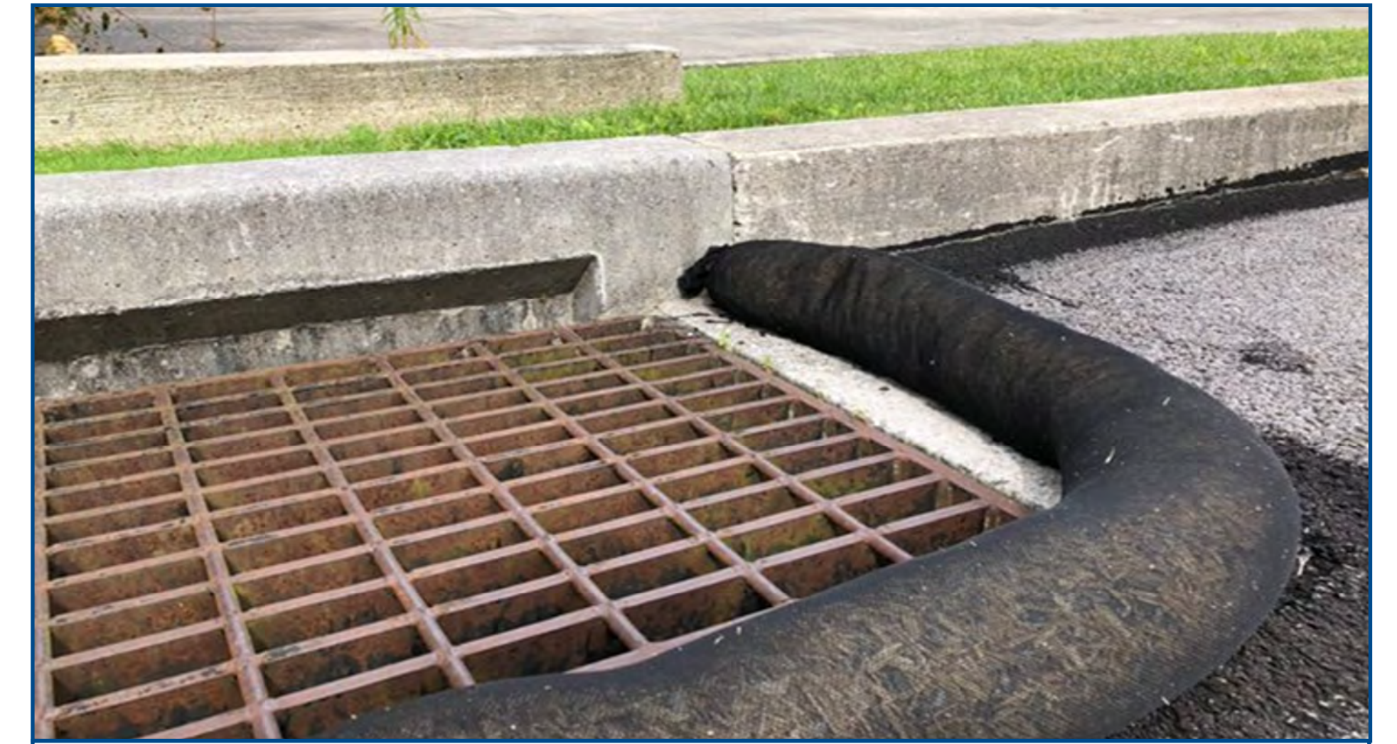
Devices such as compost filter socks are placed during construction to prevent sediment from reaching waterways.
